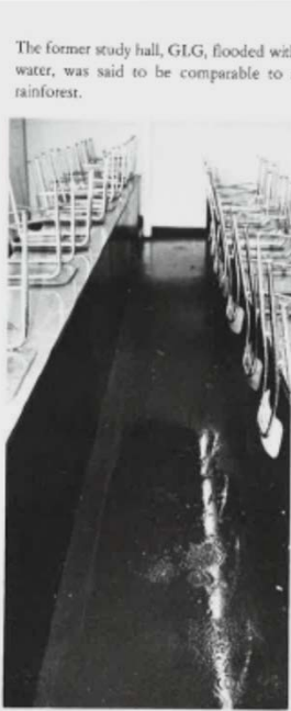
Ms. Liss's classroom lies in ruins because of leaks in the ceiling, saturating rugs that had to be removed.
